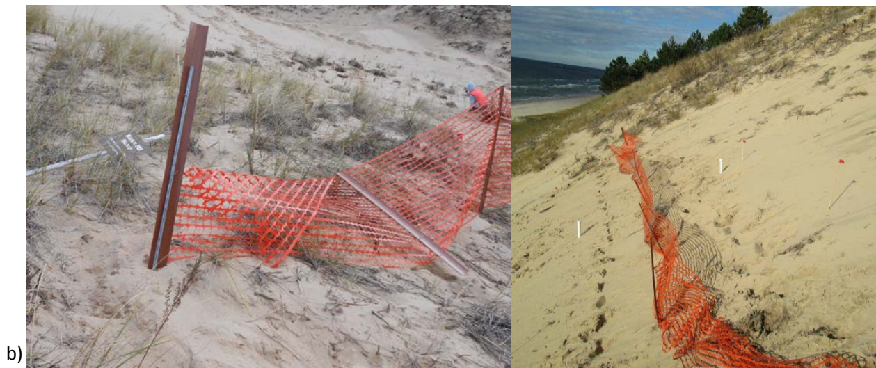
Figure 12: Although installed in April 2012, by November 2012 the sand fences already showed signs of deterioration. (a) lower sand fence (b) upper sand fence. Photos taken November 2012.
