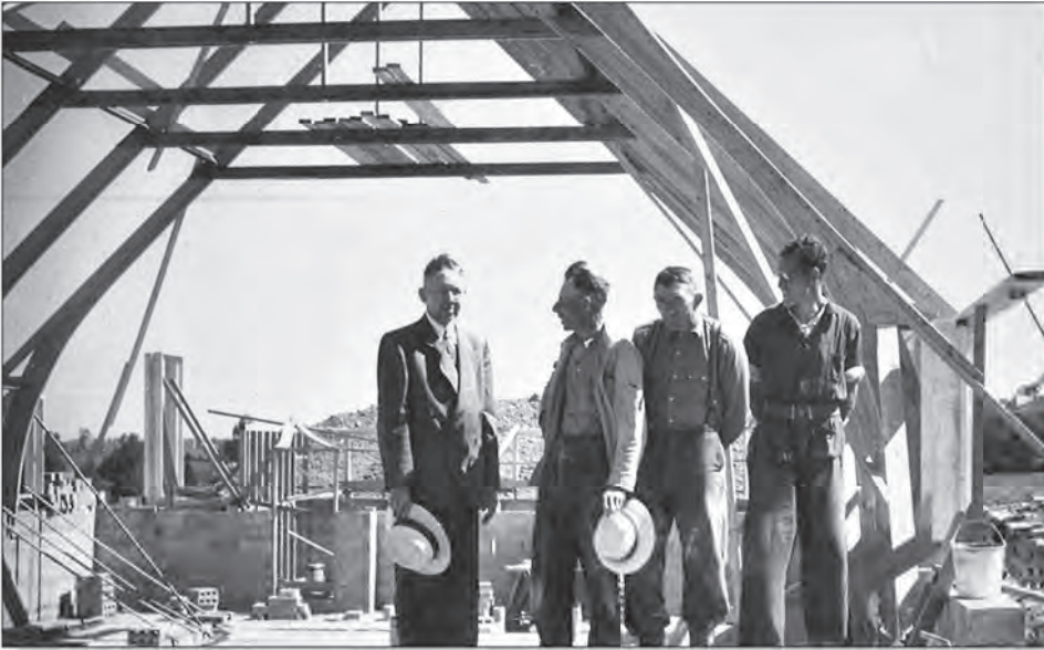
Building the first "basement" facility of Drayton Christian Reformed Church. Courtesy of Heritage Hall.
